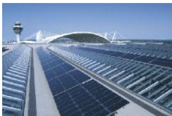
Large PV system at Munich airport. © BP Solar
